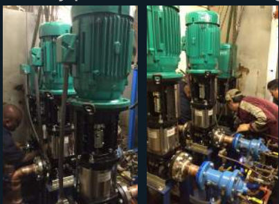
Industrial water system and cooling tower systems were replaced with new energy efficient pumps (above).
